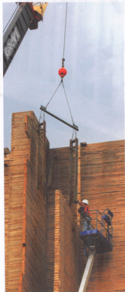
5 A pair of crane-suspended "tuning forks" are used to grasp segments of the elevator walls so they can be cut with chain saws and lowered to the ground.
