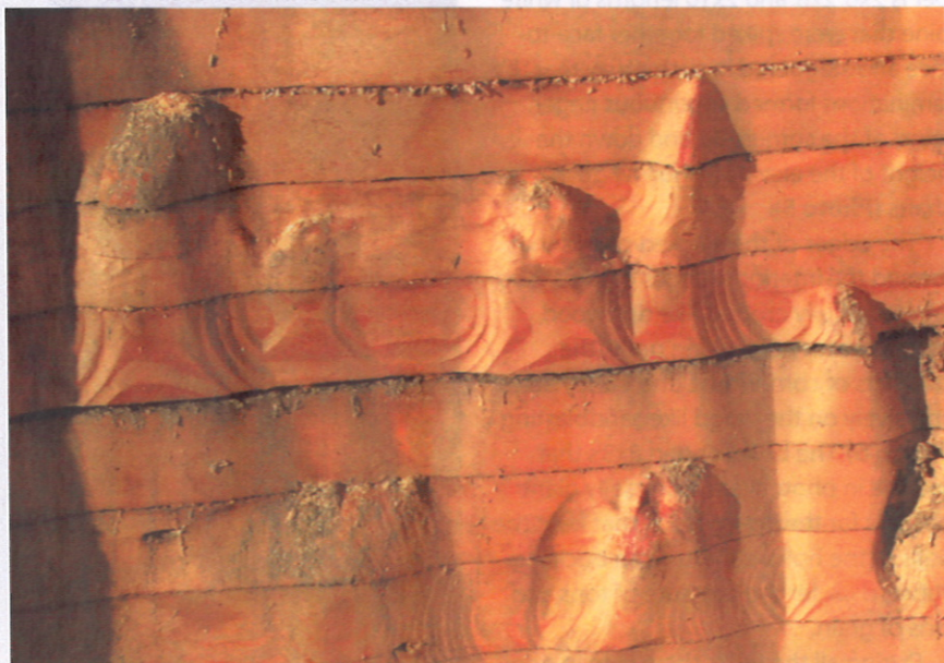
6 The abrasive, sandblasting action of grain flowing through the elevators over 100 years sculpted the interior edges of the planks. These surfaces are being saved for their unusual character.
