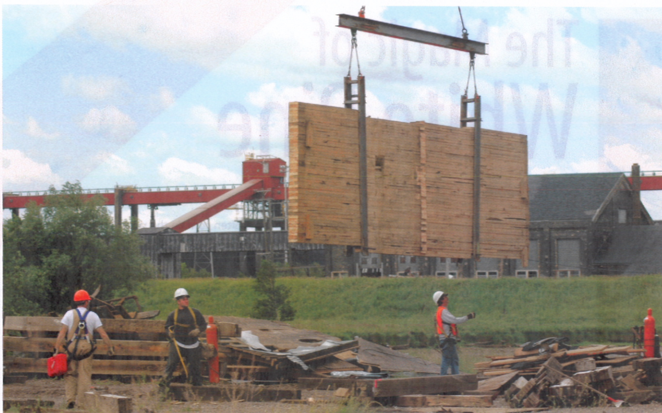
7 A small crew is working with a single crane to dismantle the three colossal elevators that made up the complex. The work is expected to take several years.
