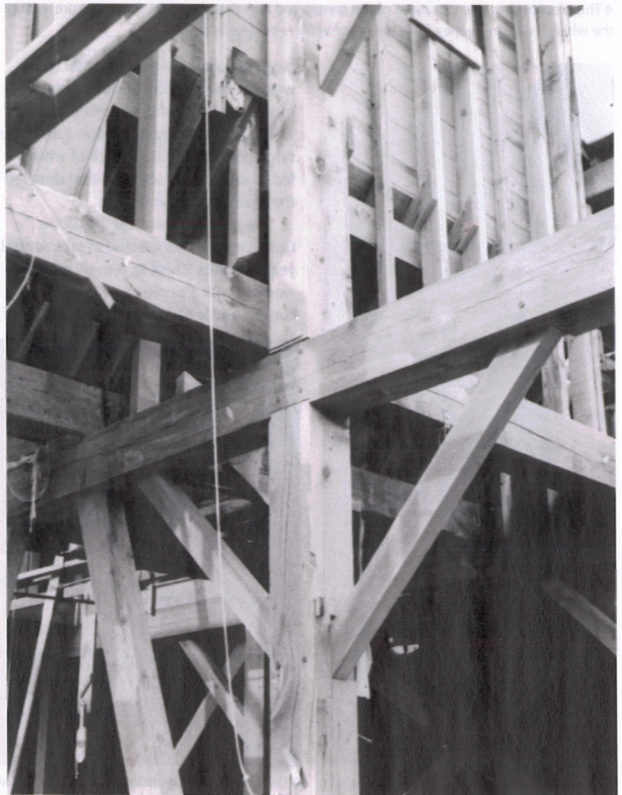
3 The ground and top floors of the elevator buildings were timber-framed with braced posts and beams.
